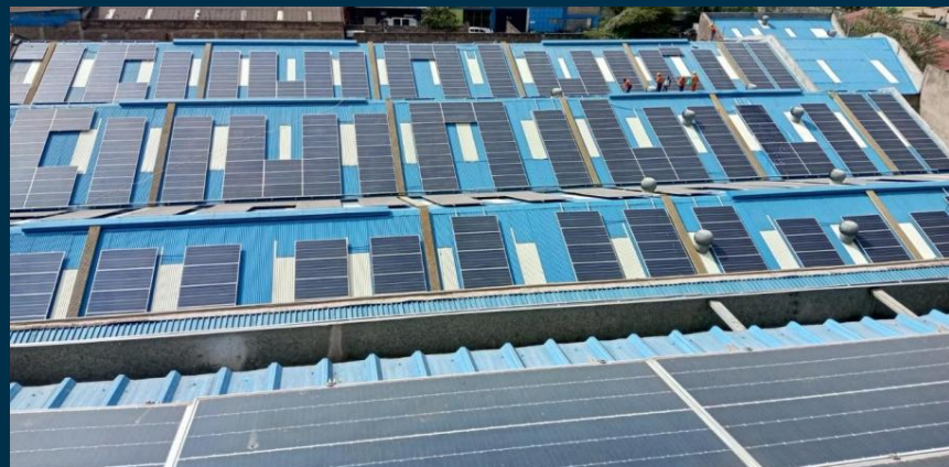
8. CHINT-SOLAR PV SYSTEM
