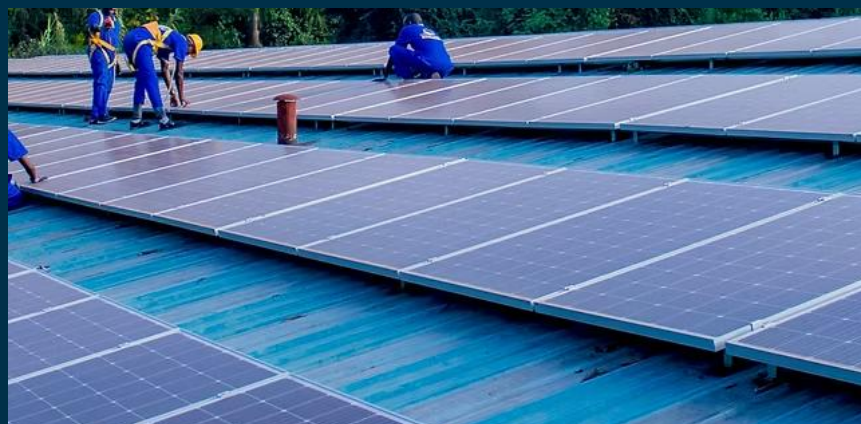
9. SCHOOL SOLAR ENERGY INSTALLATION- RWANDA
