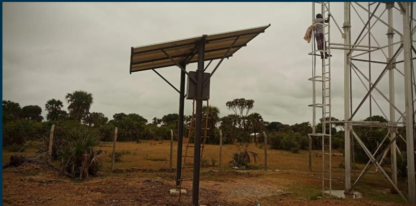
2. INGRID FARM SOLAR INSTALLATION
