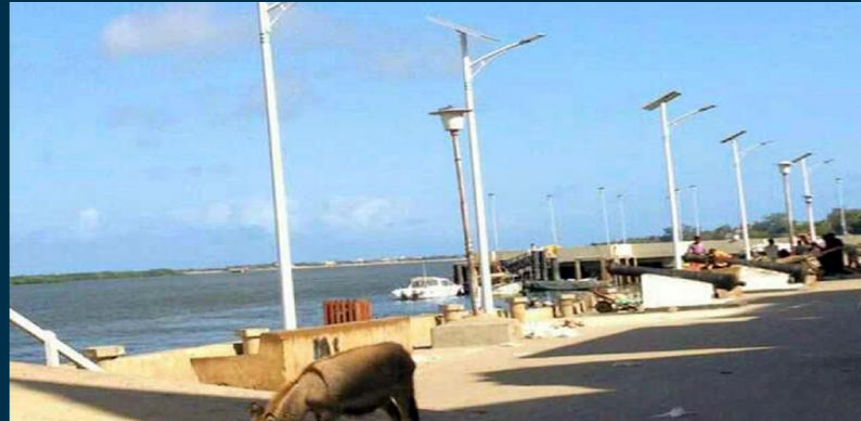
7. NEWWORLD STREET LIGHTING
